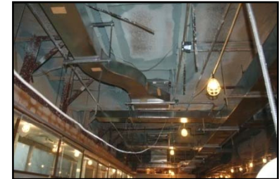
Heating, Ventilation and Air Conditioning
