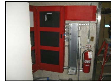
Fire Alarm System
